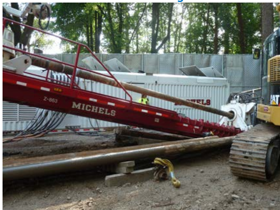
A drill rig cleans and augurs out material inside the newly installed casing at the HDD site
