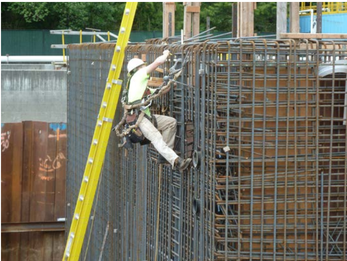
Tying rebar and preparing for a wall pour on the solids storage tank
